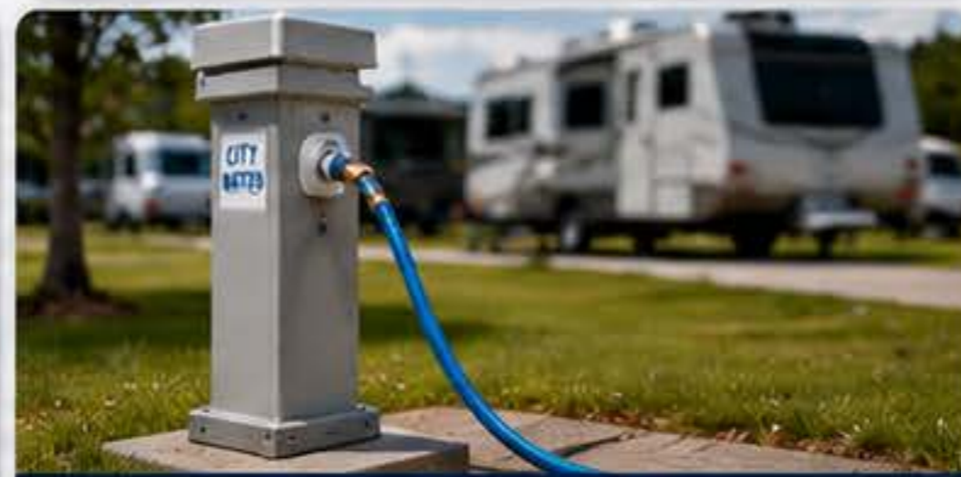
WATER HOOKUP STATION
